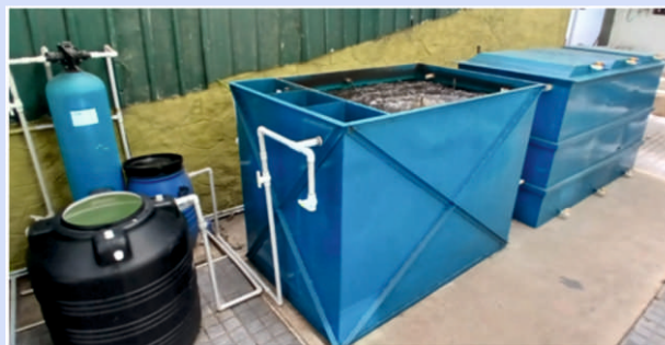
NOWA – the Decentralised Wastewater Treatment System of CSIR-NIIST
