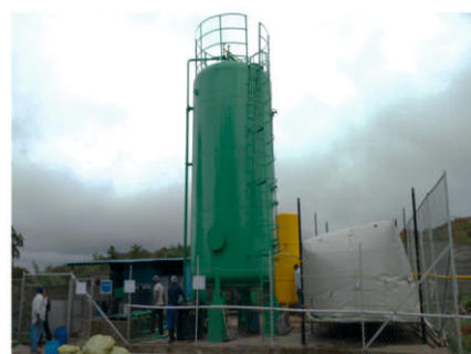
1000 kg/day Biogas plant in TAPP Kitchen at Hubli, Karnataka, India
