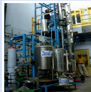
Bioaviation Fuel and Renewable Diesel Plant
